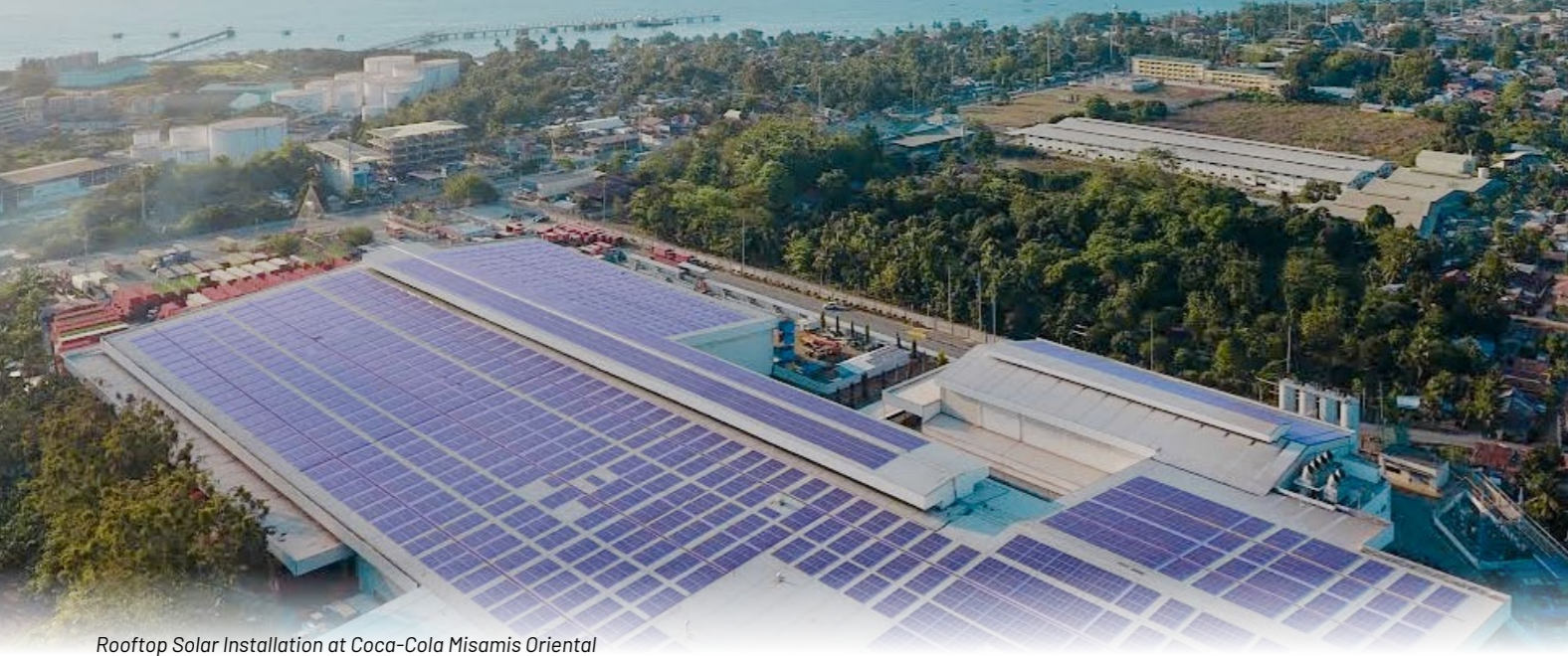
Rooftop Solar Installation at Coca-Cola Misamis Oriental
